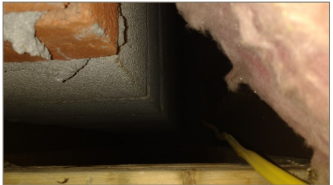
The chimney chase was implicated in air leakage.
