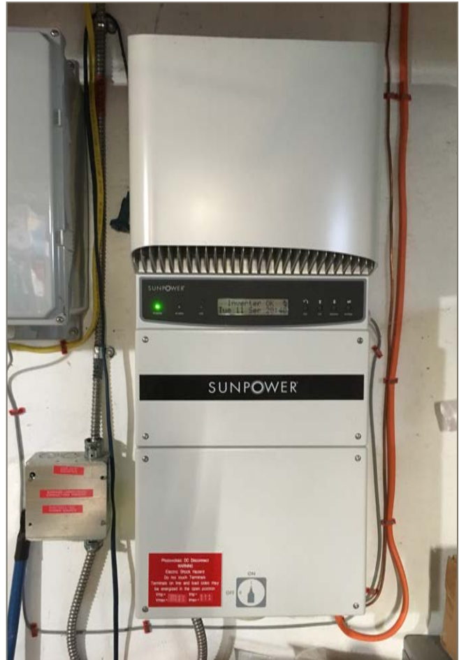
Solar panel inverter system.
